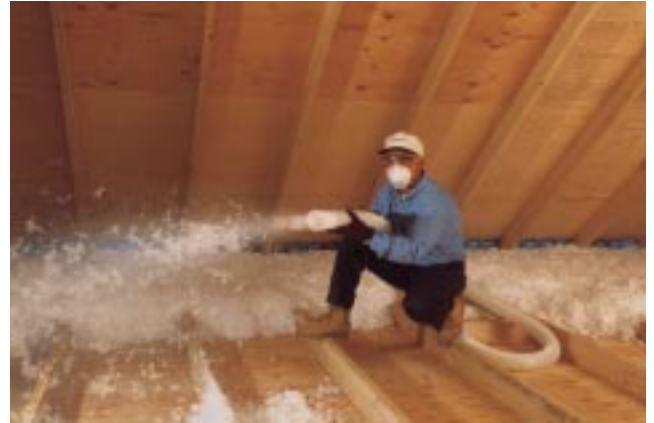
Attic insulation - photo courtesy of Certain Teed Corporation
